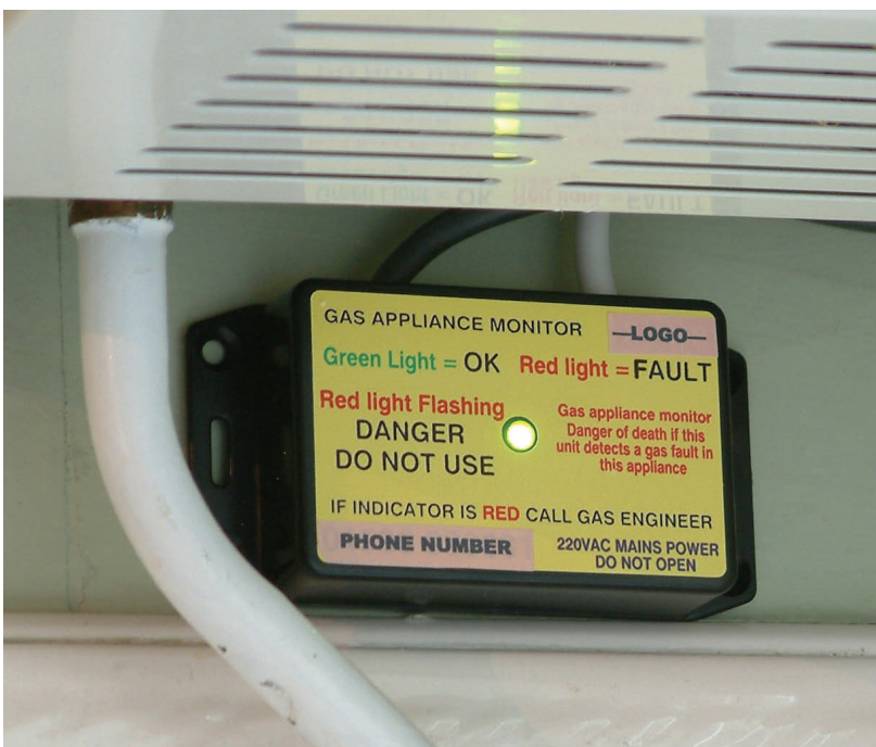
Gas appliance monitor fitted to a boiler
